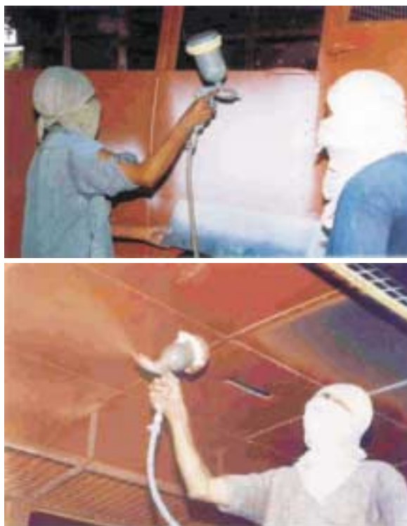
Fig. 8. Spray painters exposed to solvents and chemicals.
