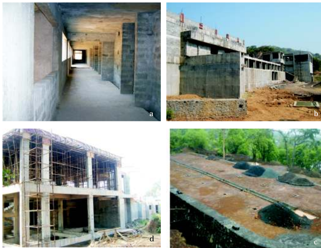
Fig.148 (a) Corridor of animal holding rooms in the Quarantine building (b) Quarantine building under construction (c) Laboratory area, operation theatre and administration sections of the Quarantine building. (d) Plynth in preparation for 16 concribs.
