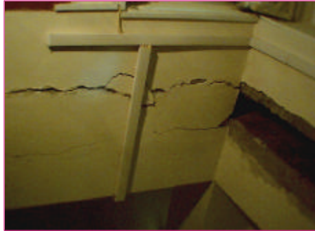
Damages sustained by the Centre's building due to the earthquake
