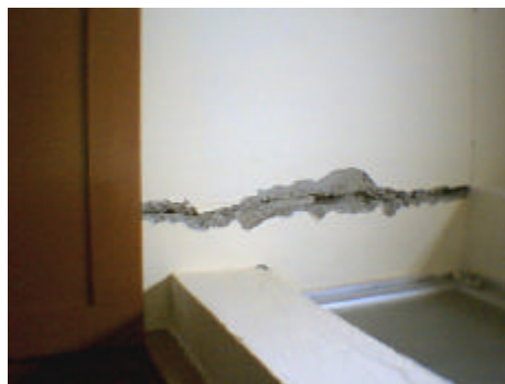
Creaks on the walls of the Centre's building
